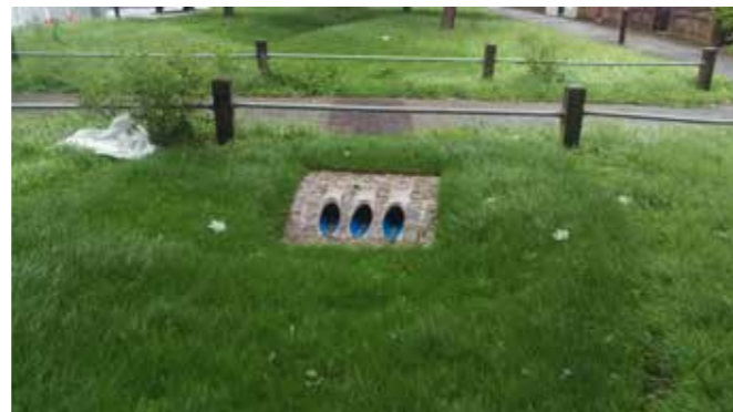
Concrete pipe surround has been used here to provide minimal cover for a driveway crossing at Devonshire Hill, Haringey.
