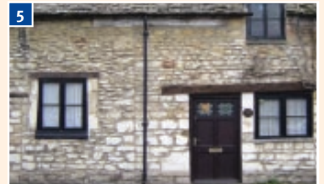
5 139 Godstow Road Grade II, former workshop dating from 18th and 19th century, coursed rubble stone with stone slate roof and timber lintels over openings
