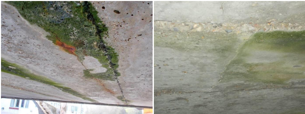
Figure 7.3 – Cracking along the plank longitudinal axis along the reinforcement bar with corrosion staining (left) and plank cracking along its transverse axis showing some deflection of concrete (right)
