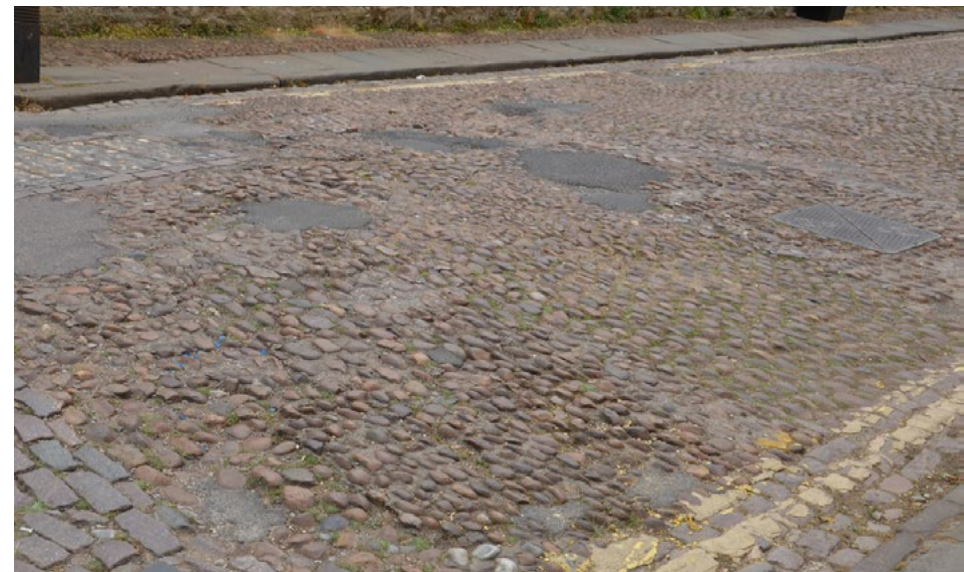
Merton Street - inconsistent materials used for repair of historic streets (OCC)
