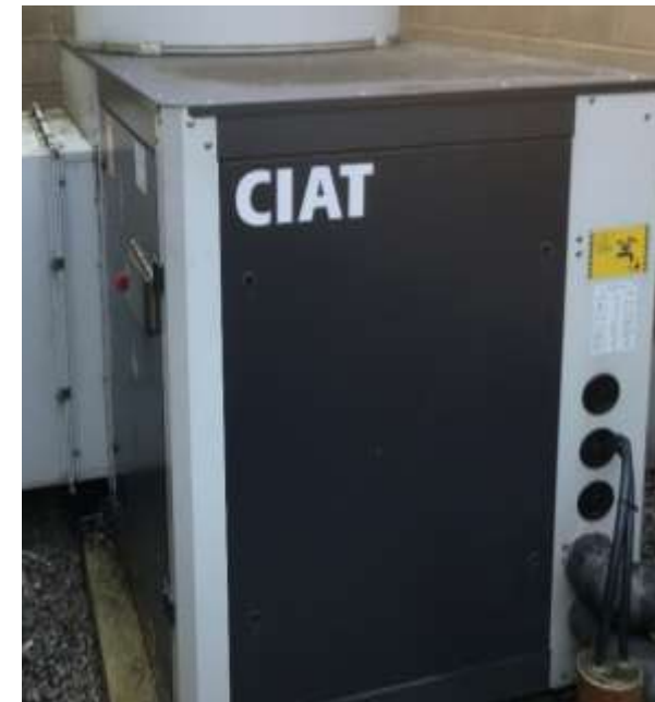
Right: Air Source Heat Pump at Wolfson College
