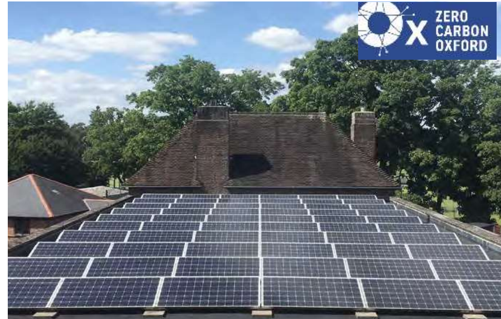
Above: Solar panels on the roof of Lady Margaret Hall
