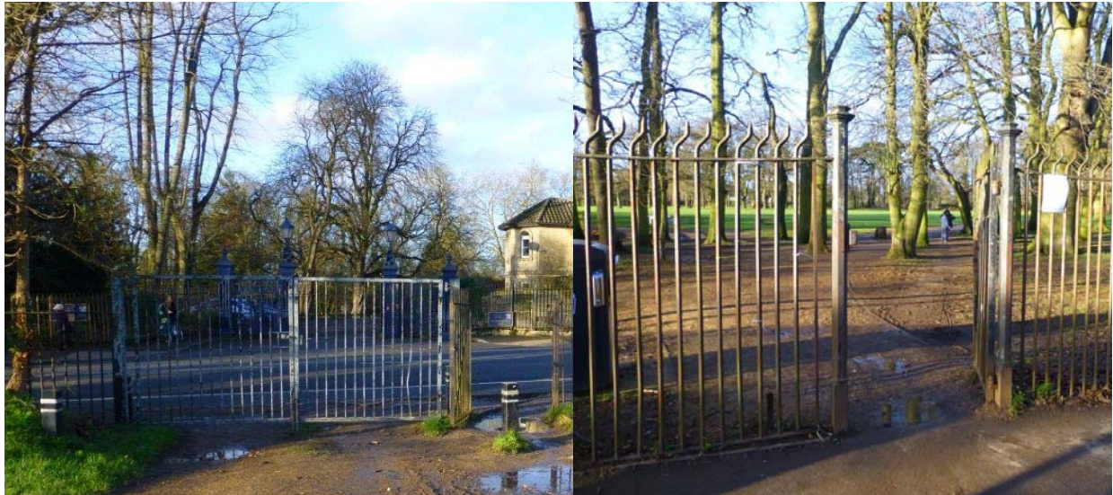
The condition and design of railings and gates is variable
