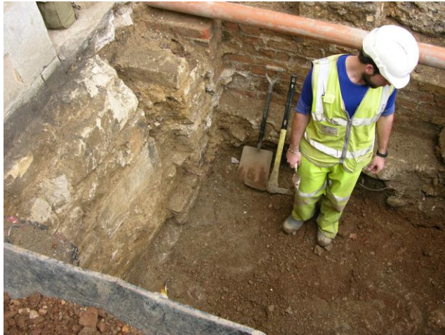
Excavations in front of the college reveal earlier wall lines and the surface of gravel walk which ran parallel to the High Street.
