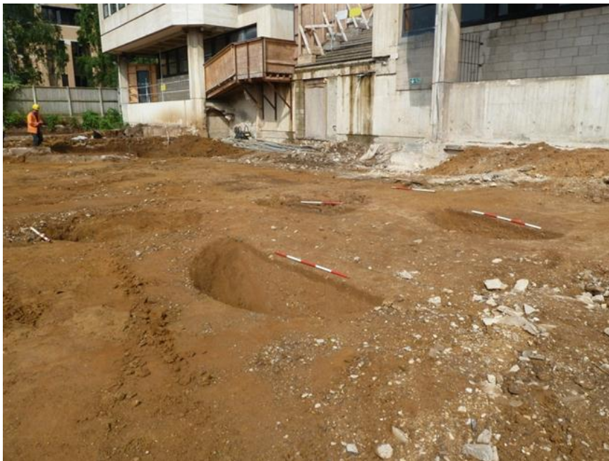
Image above: Large steep sided pits of 17th century date at the Tinbergen Building, Parks Road
