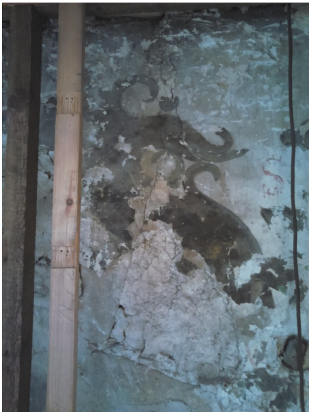
Photograph of exposed wall painting in the Stoker Room by T. Lee
