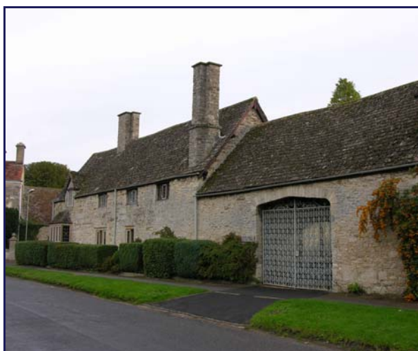
Alan Court's limestone slate roof is part of the early 20 th century refurbishment of the building
