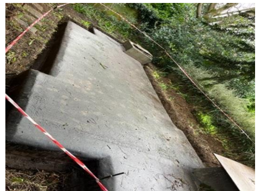
Right: the exposed top of the bunker at Chadlington Road. (Image courtesy of Wolfson College)
