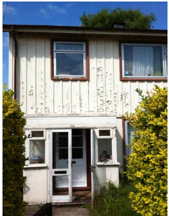
One of many steel framed, hard-to-treat houses found in the neighbourhood of Barton
