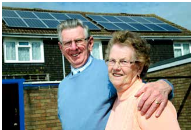
Council tenants the Parrots with their PV installation which was part of the five house pilot
