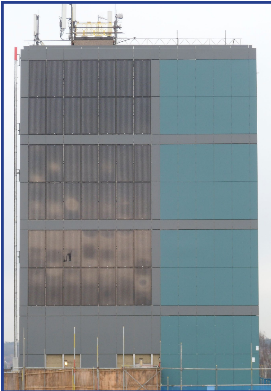
Solar PV installed at Hockmore Tower as part of the Tower Blocks refurbishment project
